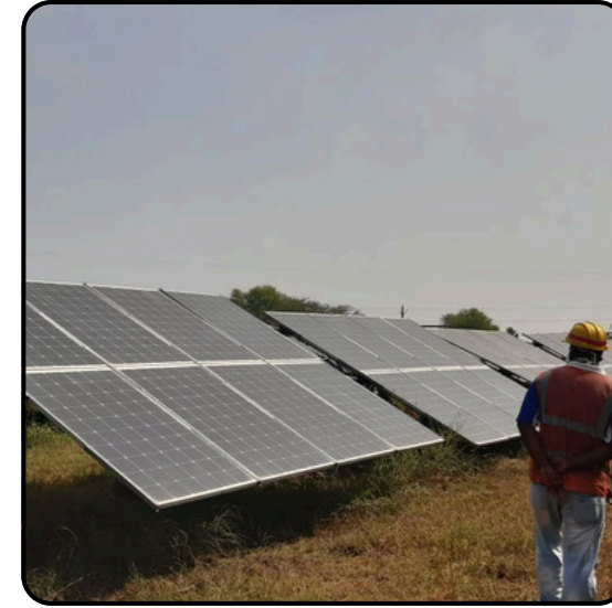
Nuvoco Vistas Corporation Ltd. (Chittorgarh, Rajasthan, India) 500 kWp
