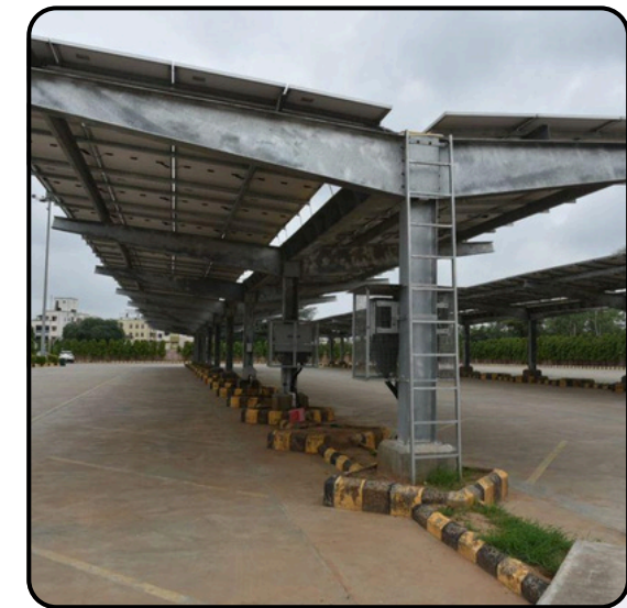
Solar Carport BAPS Akshardham (Gandhinagar, Gujarat, India) 200 kWp
