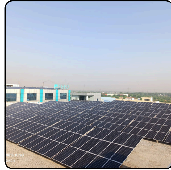
Eglo India Production Pvt. Ltd. (Rewari, Haryana, India) 500 kWp
