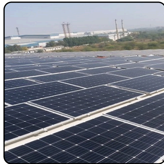
Shekhani Industries Pvt. Ltd. (Sanand, Gujarat, India) 500 kWp
