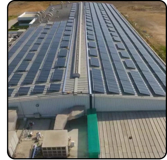
Valeo India Pvt. Ltd. (Sanand, Gujarat, India) 300 kWp
